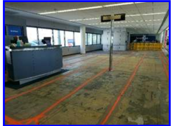
Departure gate at Rochester, NY airport being prepared for installation of phased array hearing loop.
